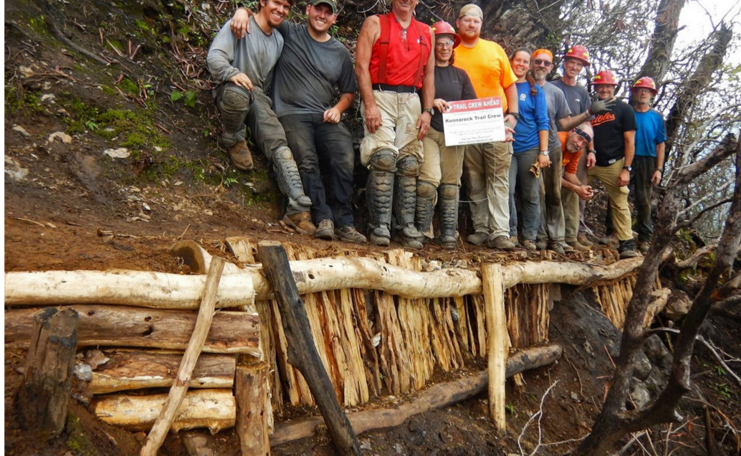
After wildfires destroyed a six-mile section of the A.T. in North Carolina, ATC's Konnarock Volunteer Trail Crew and the Nantahala Hiking Club took quick action to repair and reinforce the footpath for incoming hikers.
